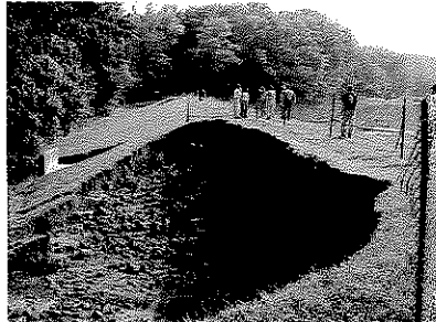
Erosion caused by floodwater overtopping the dam – a result of inadequate discharge/storage capacity.
