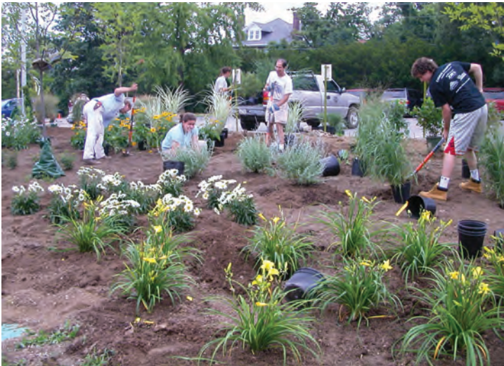
Installation of Phase II of Rain Gardens at Cincinnati Zoo proceeded under fair skies
